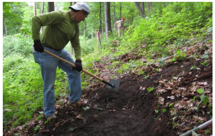
A volunteer uses a McLeod to build a new section of Hyde Park Trail south of Norrie Point.
